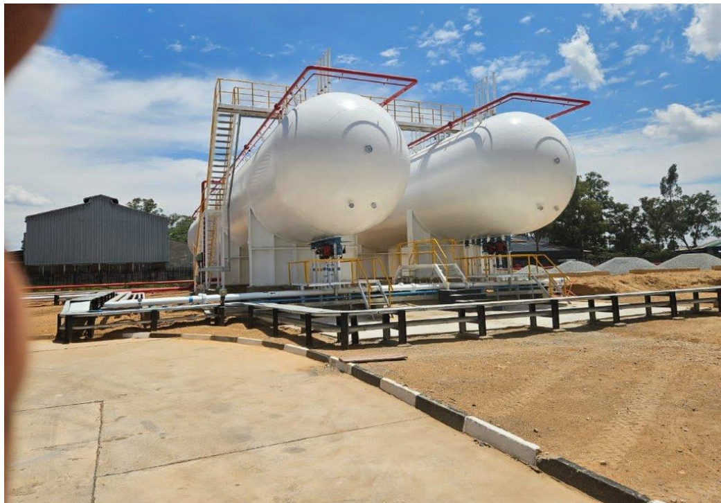
NOIC LPG Storage Depot in Ruwa
