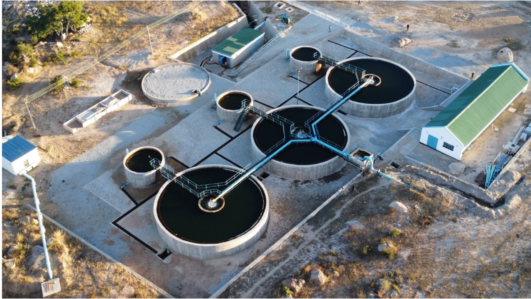
Chivu Dam Water Treatment Plant. Source: Themban Media
